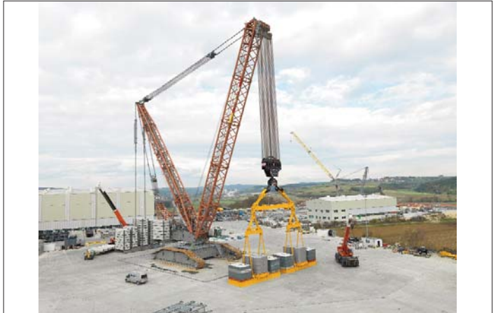
The World's Largest Crawler Crane at the Port of Indiana-Burns Harbor Photo courtesy of Ports of Indiana
